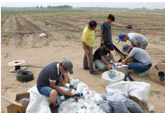
Sinofert donated and installed water-fertilizer-integrated drip irrigation system
